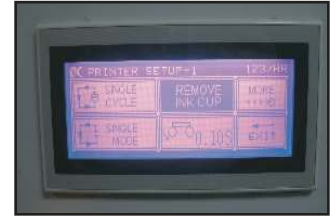
PLC control touch screen
